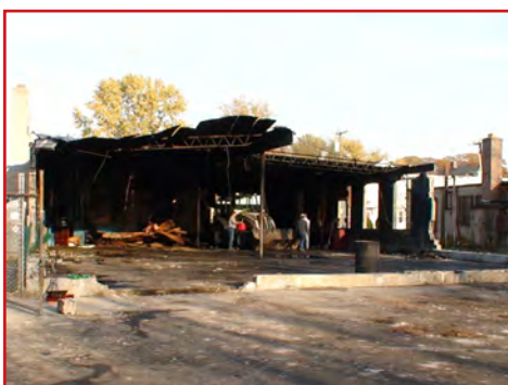
The fire completely gutted Capitol's original building, leaving nothing but a crumbling shell.
